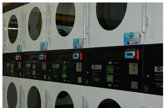
Maytag Stack 30 lb Dryers With Wireless Credit and Debit Swipe Installed
